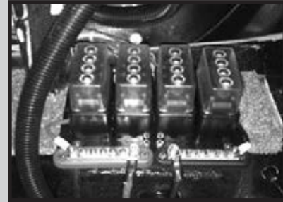
Fuse Panel - Battery Connection
